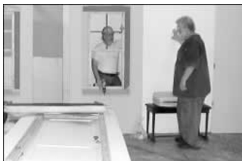
Charlie Lawson, right, holds a wall, while Hall drills in a window.
