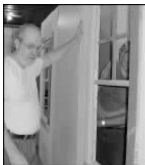
Jim Hall, left, and Clifford Cempe work on setting up the bedroom window.
